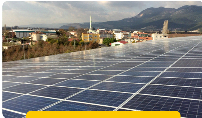
PV ROOF SYSTEM DC WIRING
